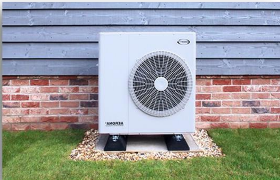
Figure 24: Air Source Heat Pump
